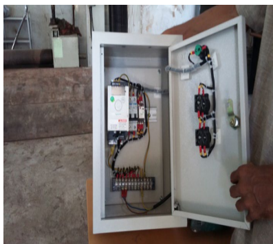
Figure 3. Vibration Control System
